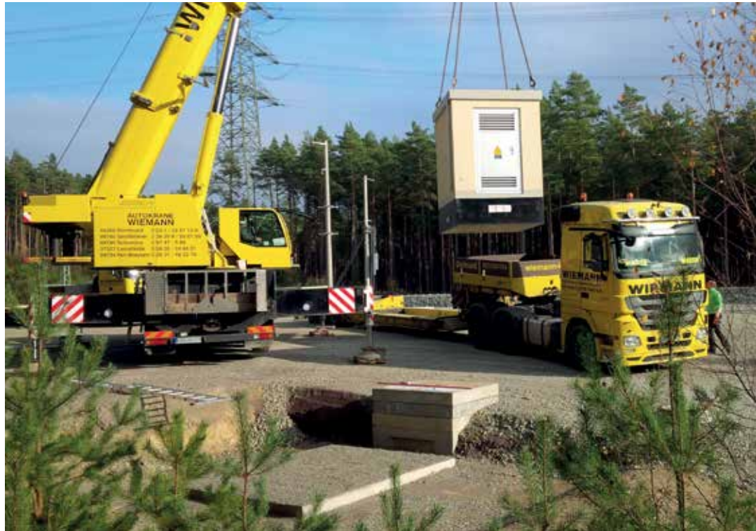
A road crane unloads one of the numerous transformer cubicles between Ebensfeld and Erfurt.
