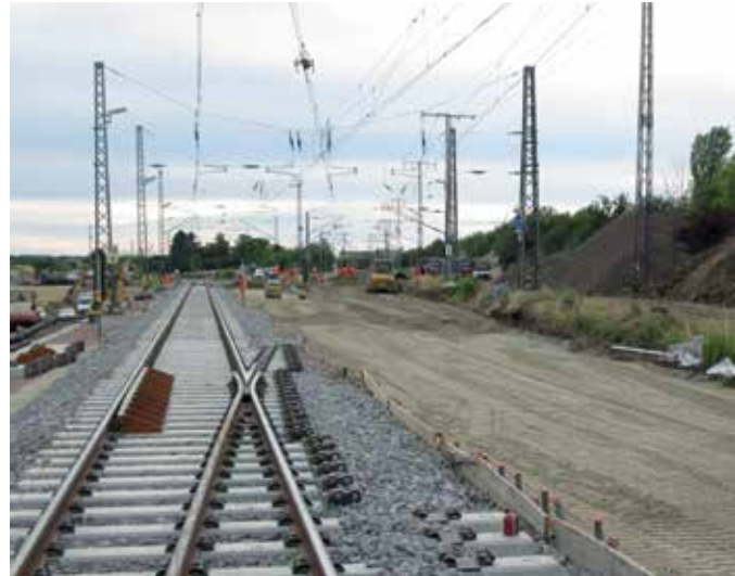
New for old: a total of nine 500 m switch points and one crossing had to be completely renewed.
