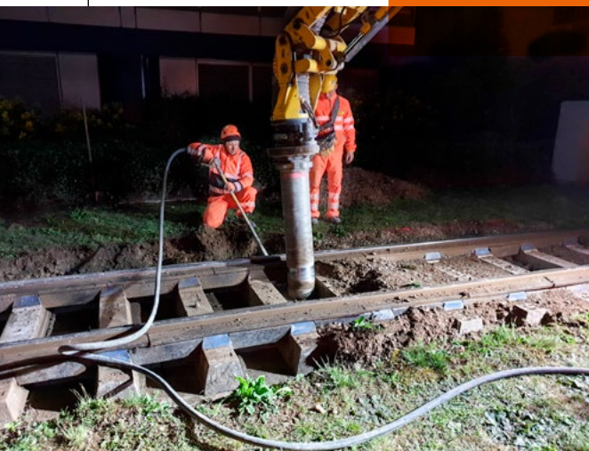
■ Exposure of the track supporting layer on a private line (ballast and grass)
