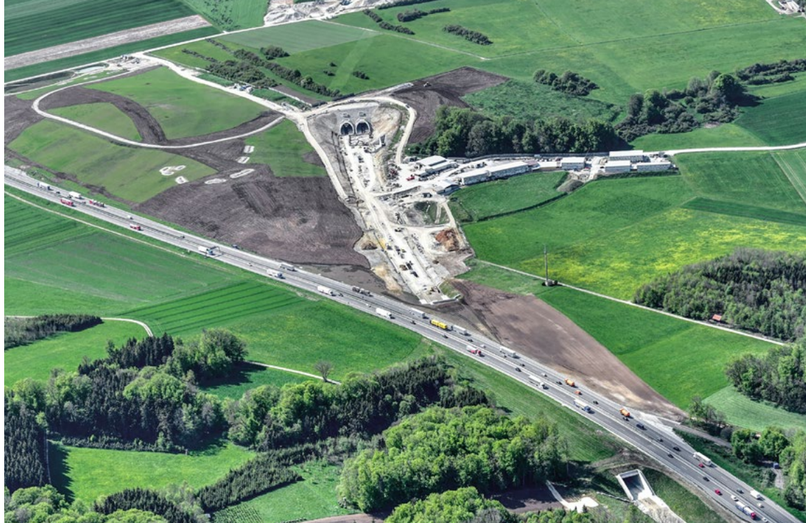
■ The Joint venture construction office at the eastern mouth of the Steinbühl Tunnel
