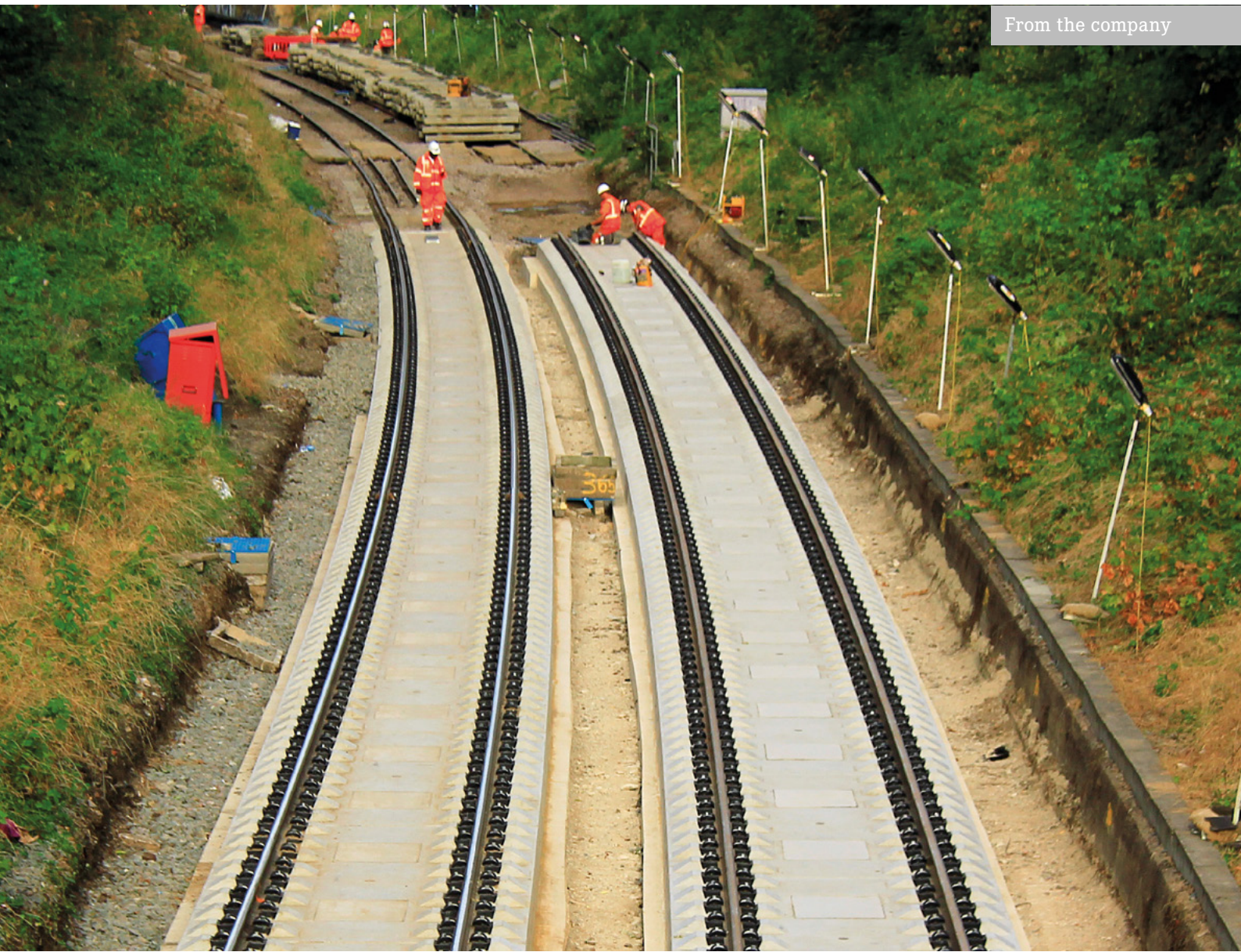
The fourth slab track project: installation of slab track at Gospel Oak.
