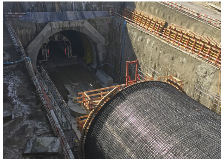
Simply efficient: MyNet facilitates the handling of large and complex projects such as the Rosshäusern tunnel
