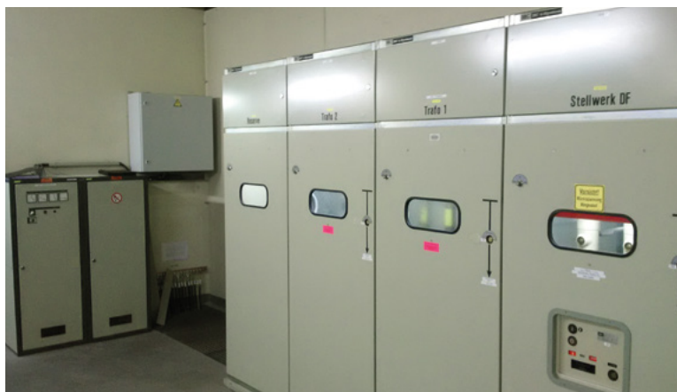
Arrived: the new transformers at Düsseldorf main railway station.
