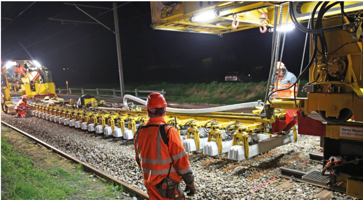
One of the tasks involved in mechanised track construction: placing the concrete sleepers to which the new rails are attached.
