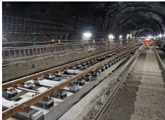
Installation of slab track in the two-track tunnel at Queen Street railway station
