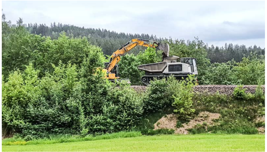
Ballast works by tracked excavator and dumper during the construction project in Zwiesel
