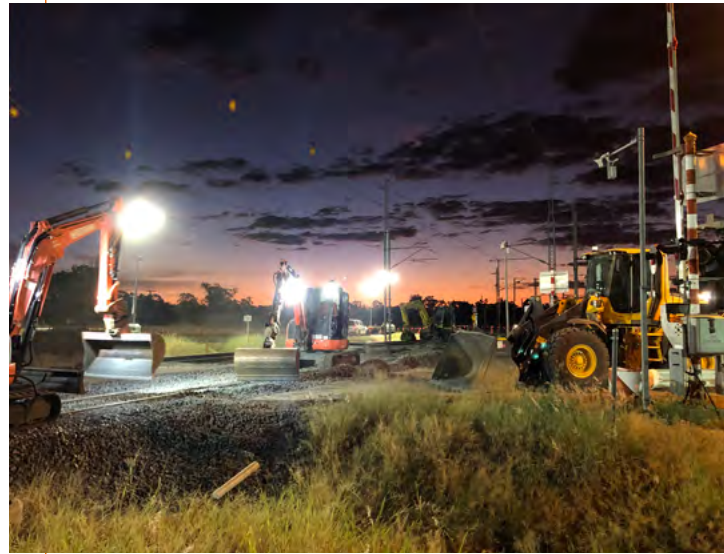
2x 5T excavators work together with loaders to fill and pack the ballast before renewing the track.
